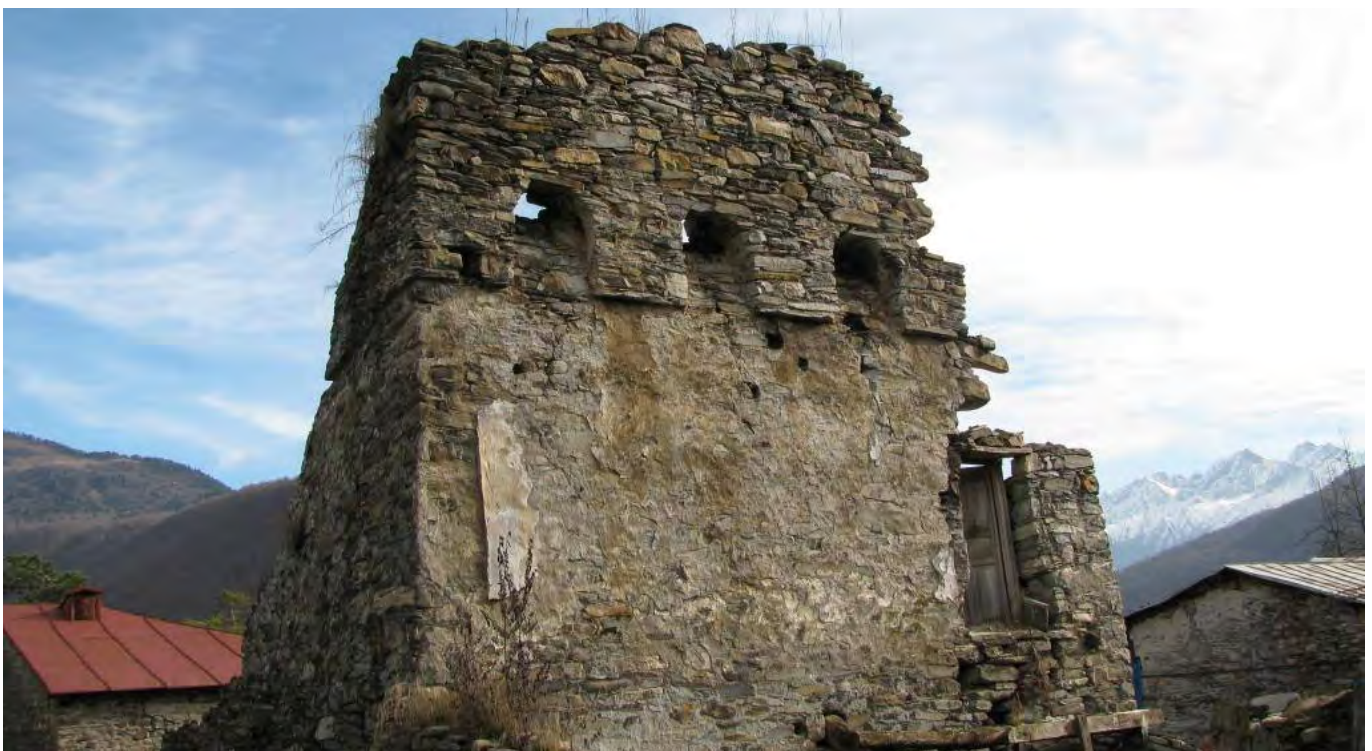
"Duroiani Sakhli", a traditional tower house in village Ghebi, Upper Racha, Gerorgia, 2019.
